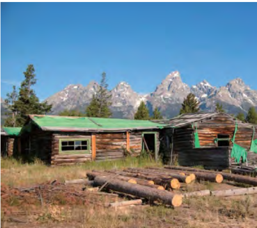
Performance Assessment and Evaluation of Hydrophobic and Ultra-violet Protective Treatments for Historic Log Structures , Courtney Magill, 2015
